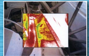
Moisture intrusion into deck core at forward of port deck winch.
